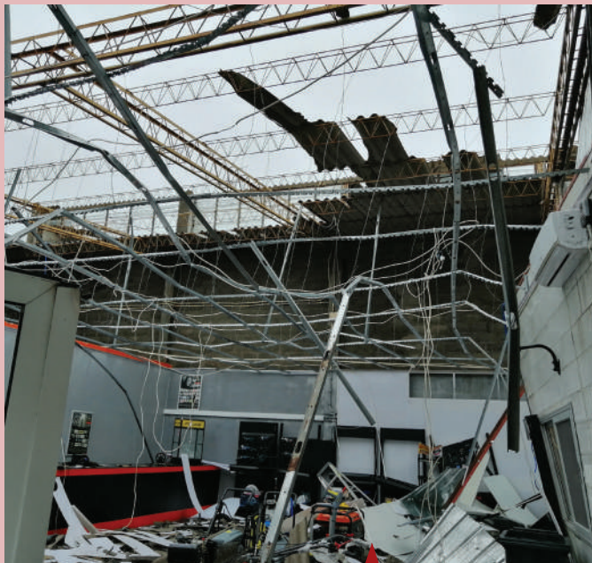
BMG (Bearing Man Group) facilities totally destroyed
